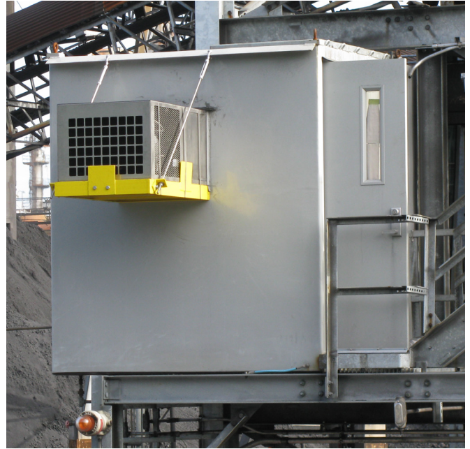
NEC Class II Division 1 Unit Cooling and Heating at Coke Processing Plant
