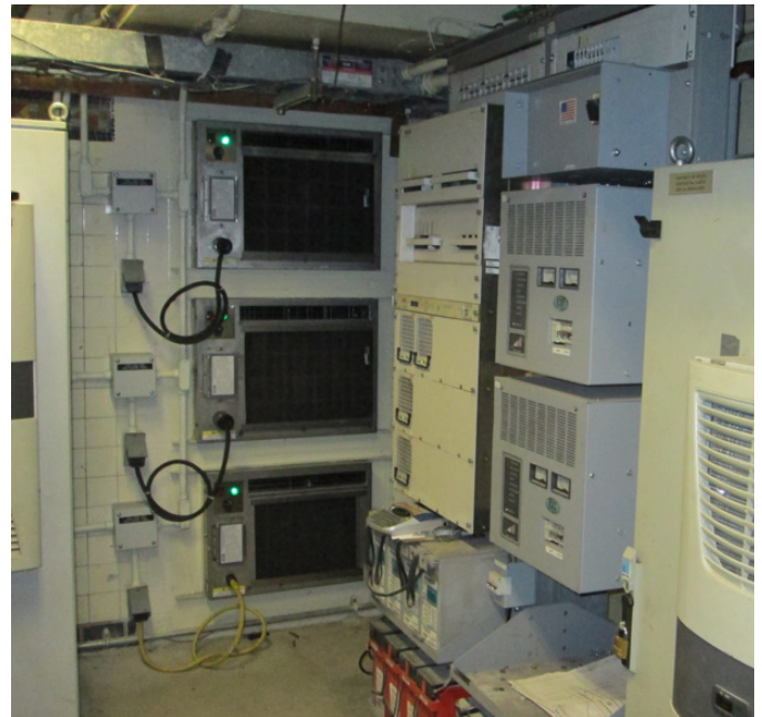
Underground Control Room
