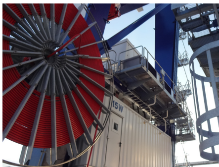
Units Installed At A Global Terminals Factory
